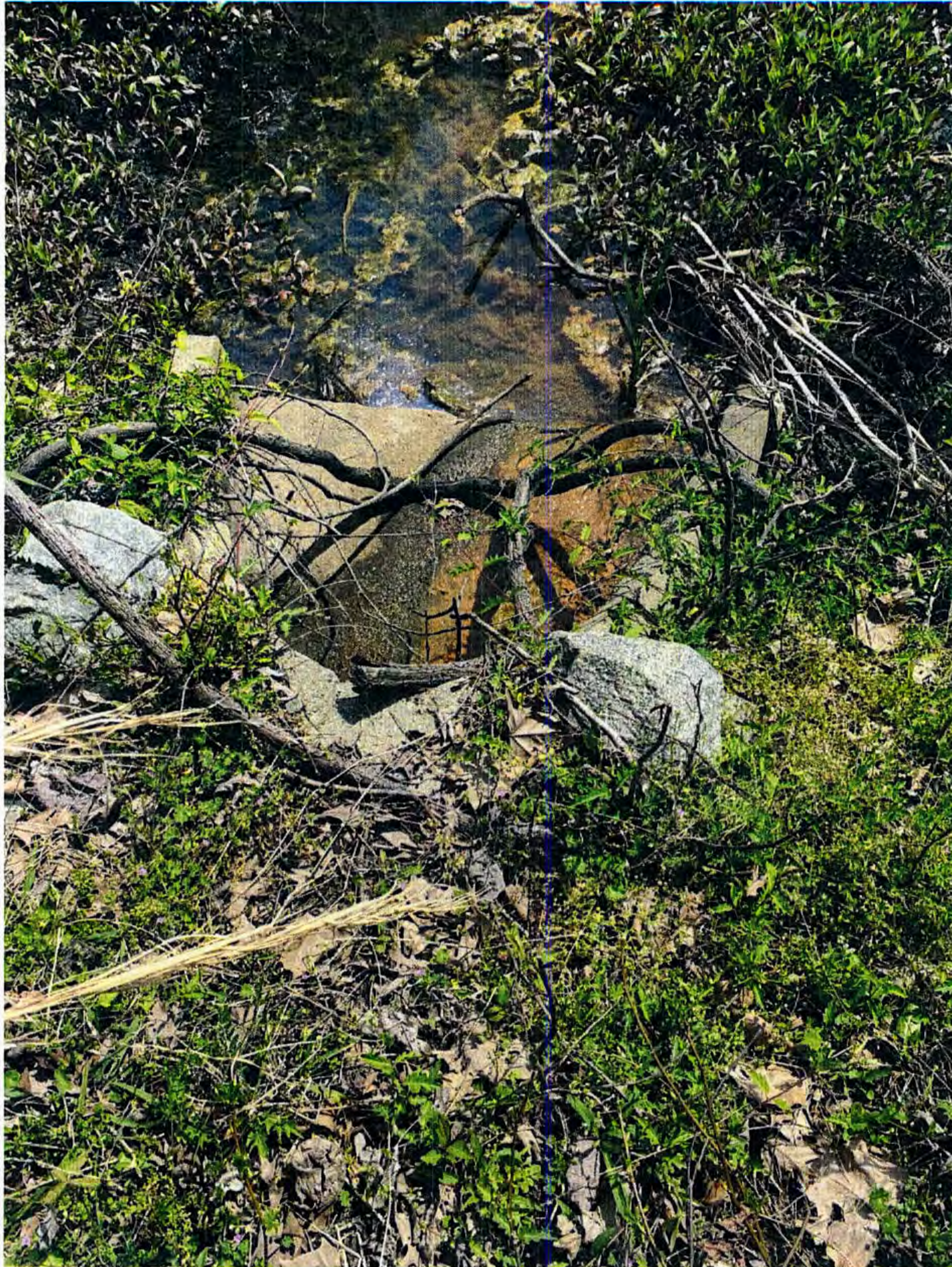
Photo #OF-G-1. In flat area of pipe end section – accumulated orange deposits/stains similar to pavement staining color near dumpster.
