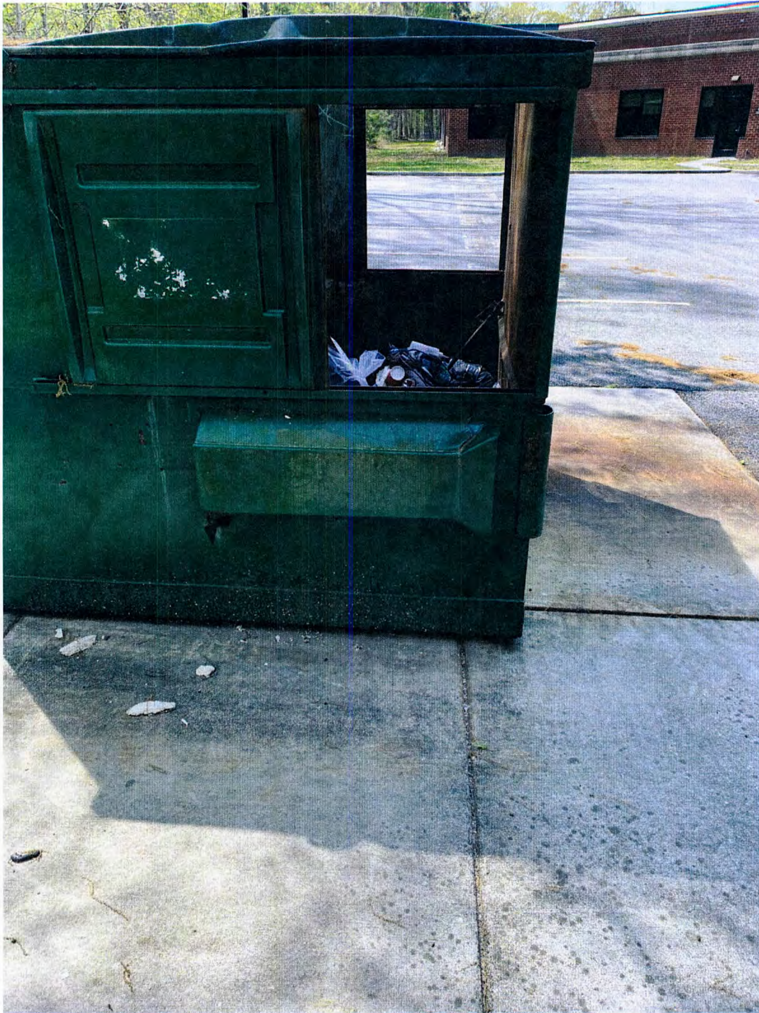
Photo #OF-G-3. Staining apparent on pavement all the way to receiving inlet (see also 2019-2020 report for this outfall). Staining indicates leak(s) in the bottom of dumpster. Dumpster also observed to be open, allowing for exposure of contents to stormwater.
