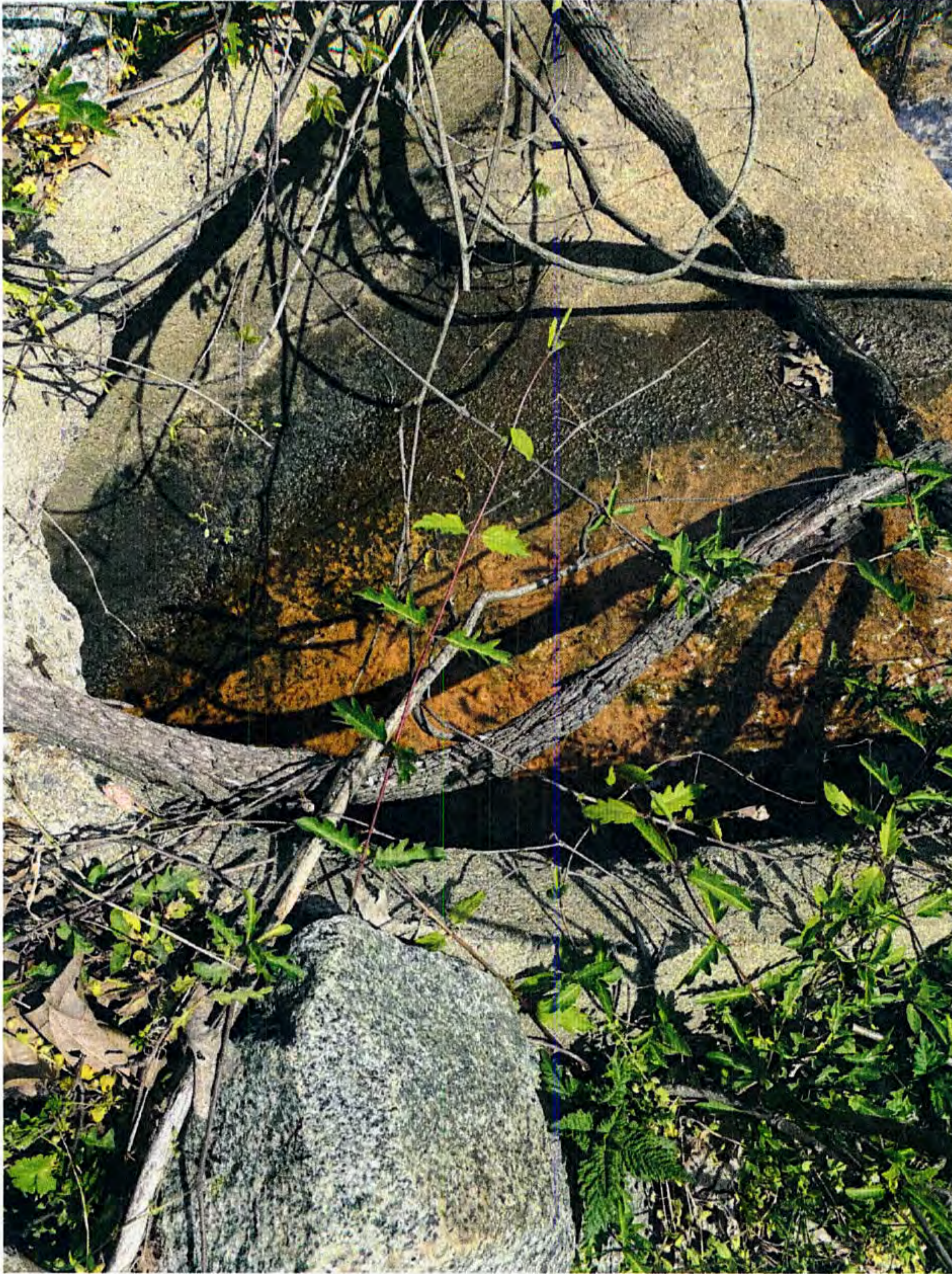
Photo #OF-G-2. In flat area of pipe end section – accumulated orange deposits/stains similar to pavement staining color near dumpster.
